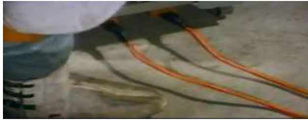
Check primary circuit wiring connection
